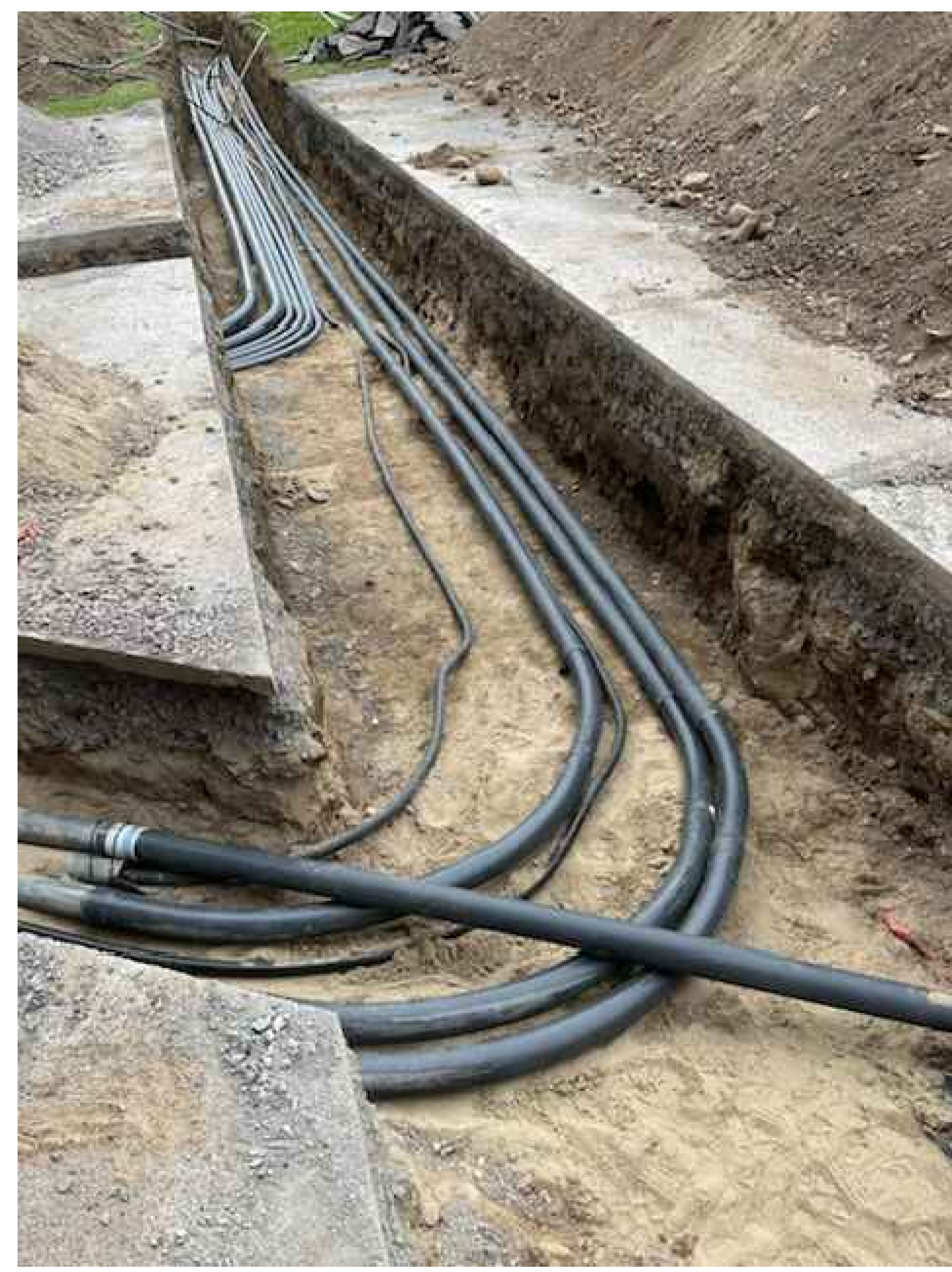
3 EXISTING UNDER GROUND CONDUITS FROM BASEMENT ELECTRICAL ROOM TO PORTABLES E1 N.T.S.
