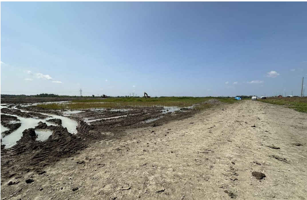
Photograph 4: View of southeastern portion of the Phase I Property that better highlights the western edge's grading.
