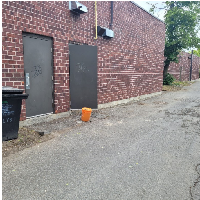
Photograph 4: View of the back of the on-site dry cleaner (open door), view is looking southwest. A monitoring well was observed behind the dry cleaner unit, while a catch basin was visible to the northwest of the dry cleaner.
