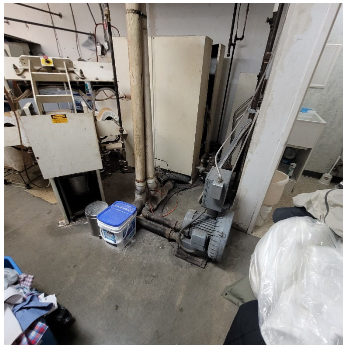
Photograph 6: View of the dry cleaning equipment on the interior of the dry cleaner unit. View is looking west.
