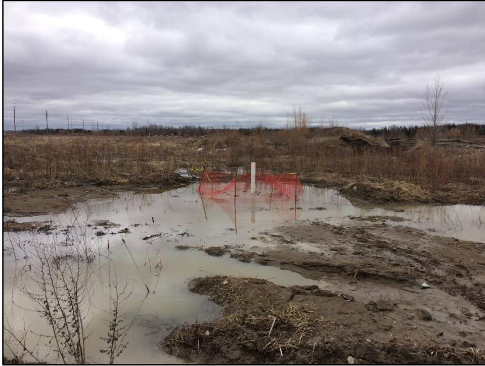
Photo 1: Standing water near Test Fill Pile D in April 2017.
