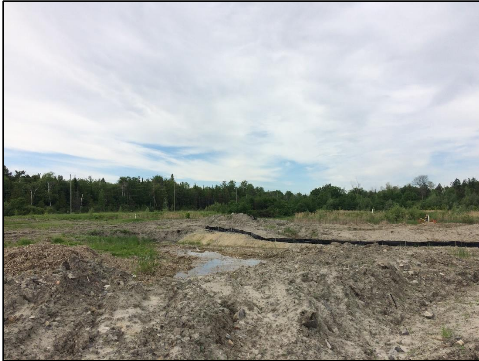
Photo 3: Soil berms and standing water within south portion of HMB West in June 2017.
