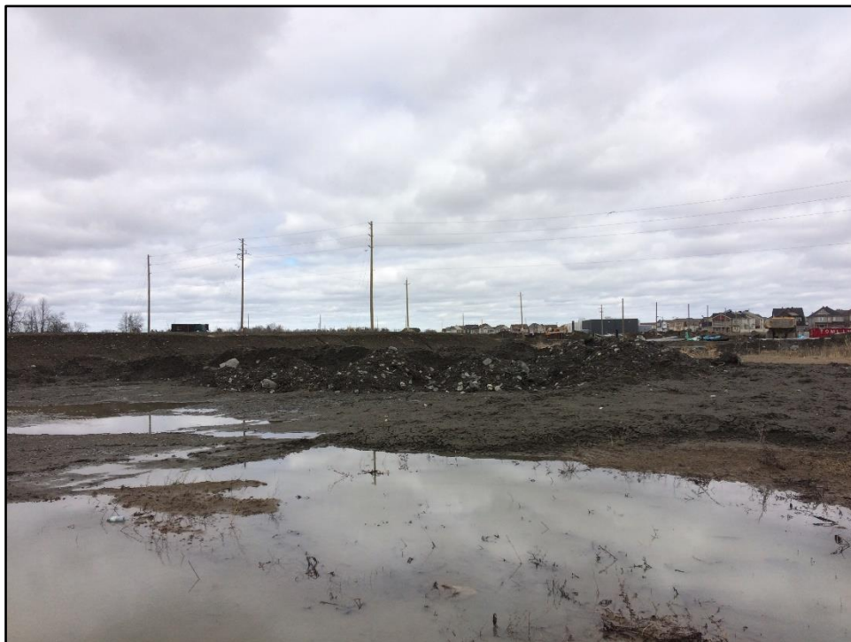
Photo 2: Standing water in east portion of Half Moon Bay West in April 2017.
