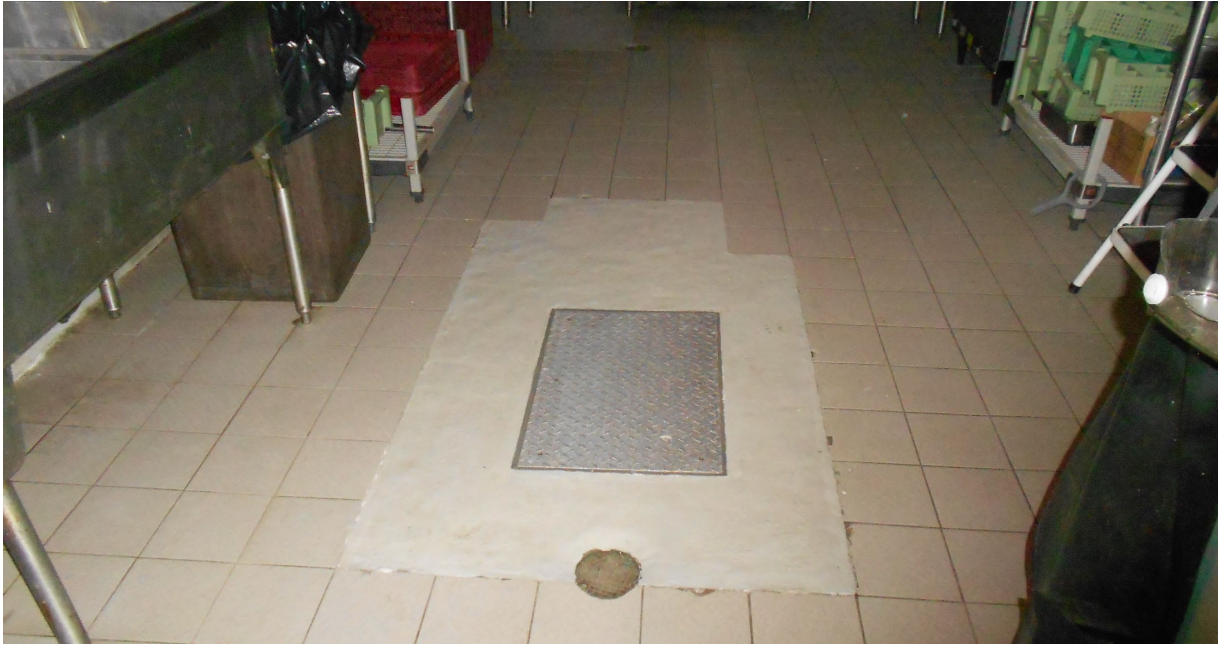
Photo 21 View of grease trap in kitchen of the Corporate Building.
