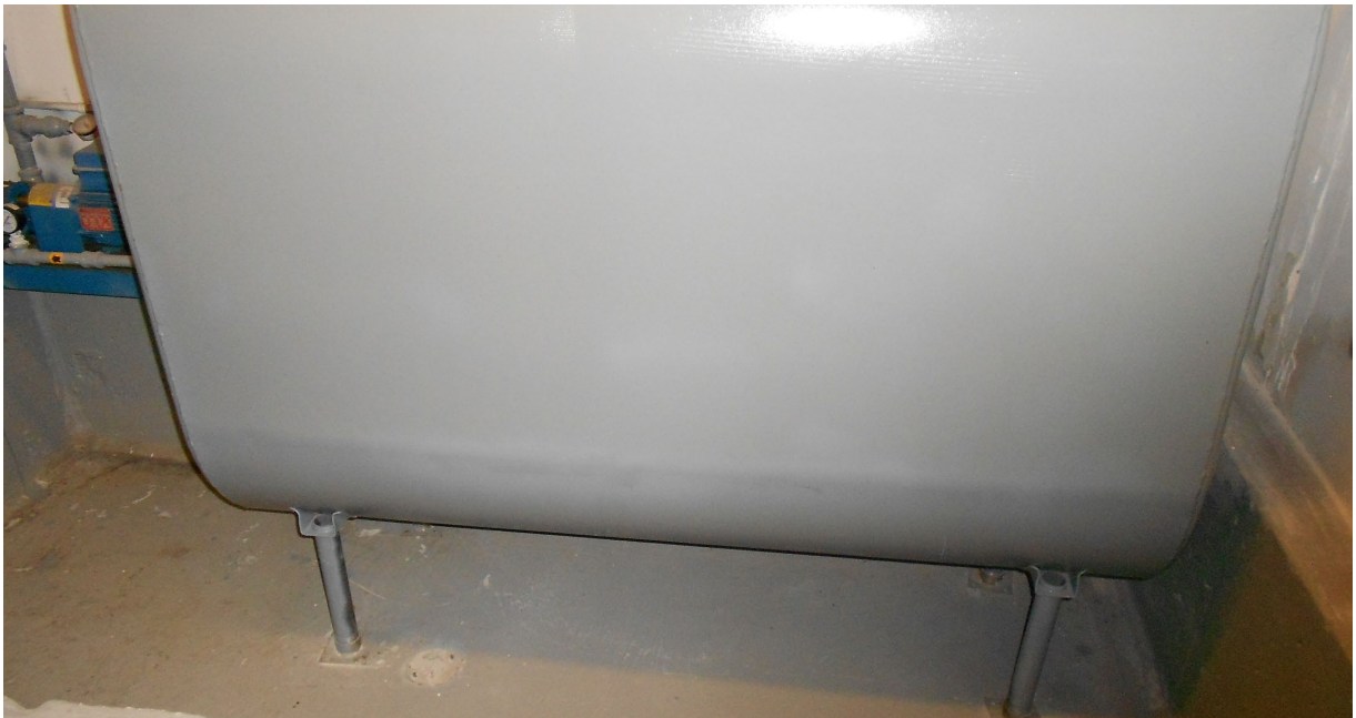
Photo 20 View of bulk diesel tank on ground floor of Tower 3 (feeds day tank located in Tower 3 penthouse).
