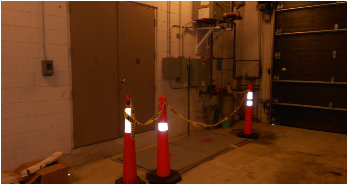
Photo 22 View of sump pump pits and glycol system for Tower 2 basement loading ramp with trench drain.
