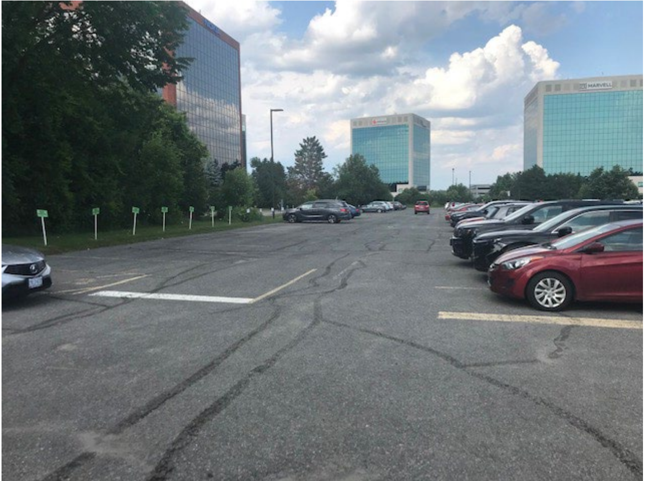
Photo 3 View of northern end of Site (parking lot), facing east, adjacent to Nokia Office Complex property to the left.
