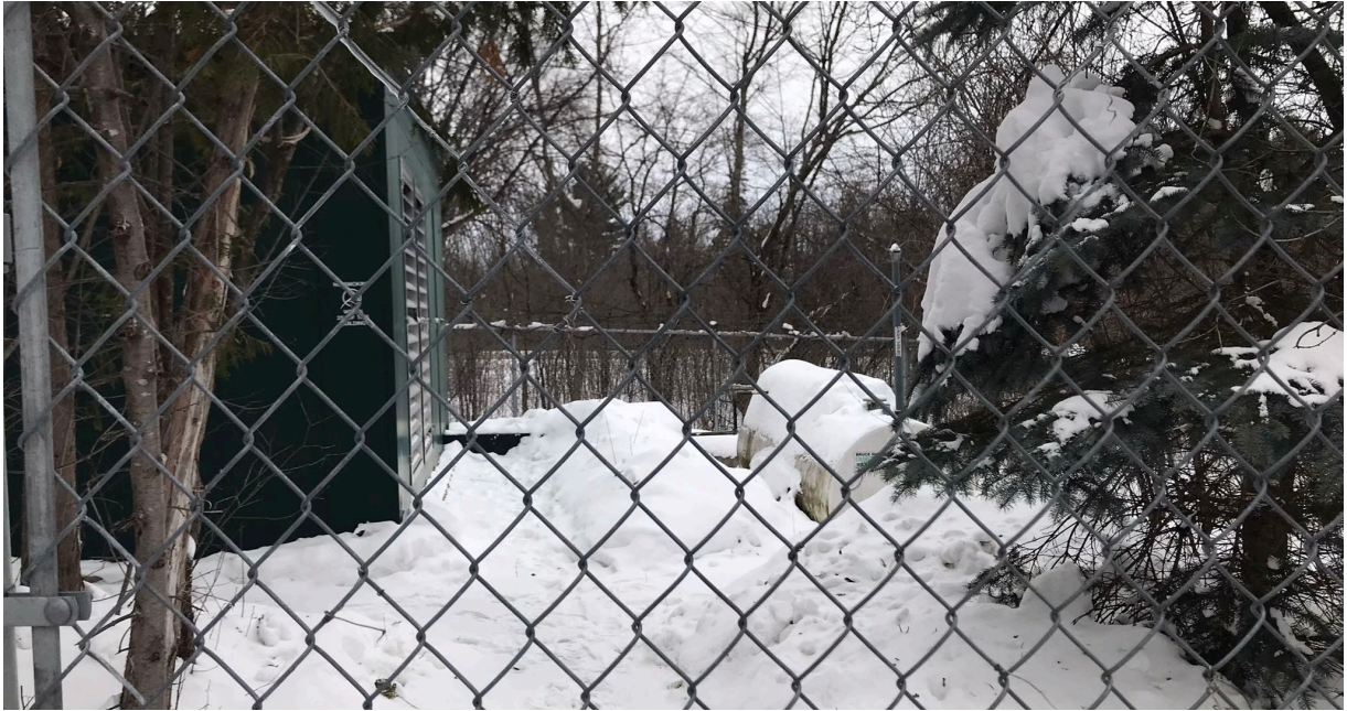
Photo 7 View of Diesel Generator building (left; decommissioned flat tank below generator) and diesel tank on exterior (right), facing east.
