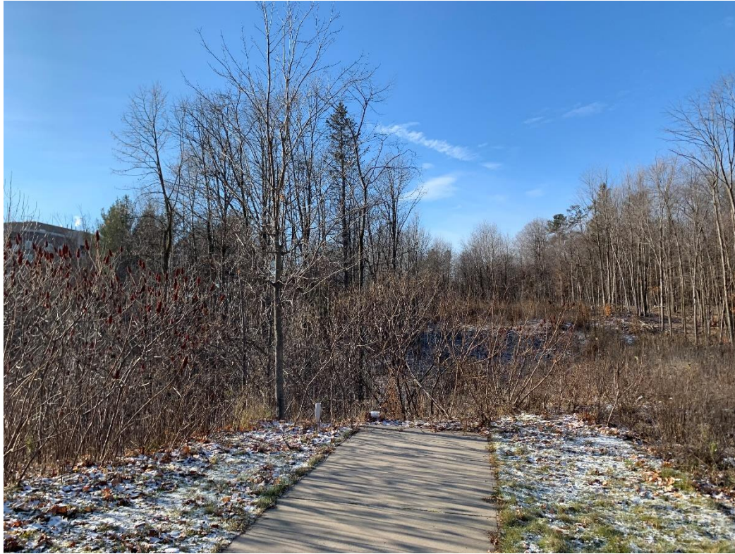
Photo 13: Concrete sidewalk located east of the northeastern portion of the Site, along Canadian Shield Avenue.
