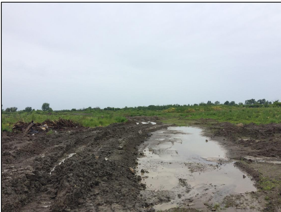
Photo 4: Standing water with fill and debris piles in central portion of HMB West on June 29, 2017.
