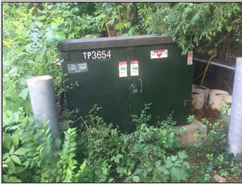
Photo 9 – Pad-mounted transformer located on the east portion of the Phase One Property.
