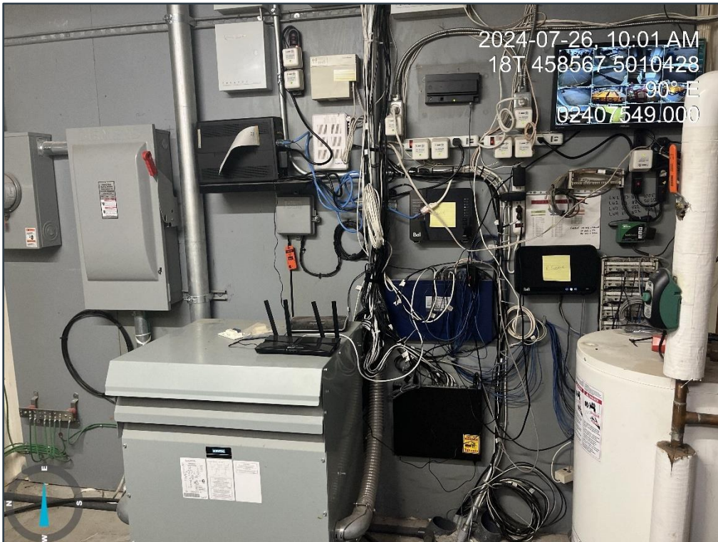
Photograph 6: Electrical Room located in the Staff Room (6622 Bank Street).
