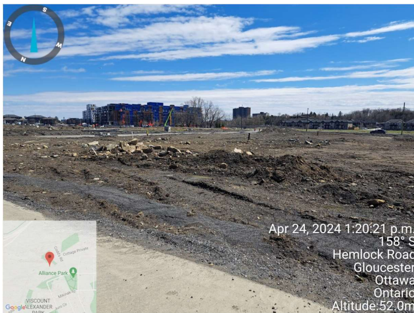
Standing at northwest side of Street No.1 and looking towards southeast of Block 5 : No indications of existing slope greater or equal to 2 m in height or any settlement. Presence of a pile of concrete block pieces.
