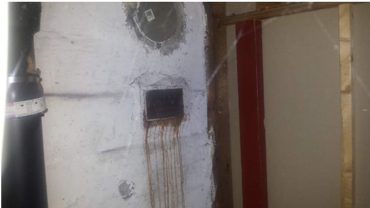
Photograph 8: Chimney cleanout at basement of 398 Roosevelt Avenue.
