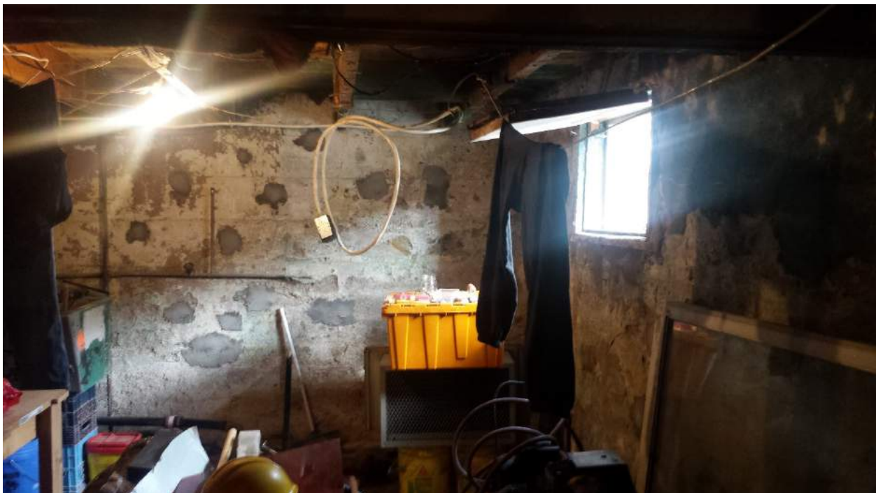
Photograph 4: The basement of 406 Roosevelt Avenue, showing the reported former location of the fuel oil tank.
