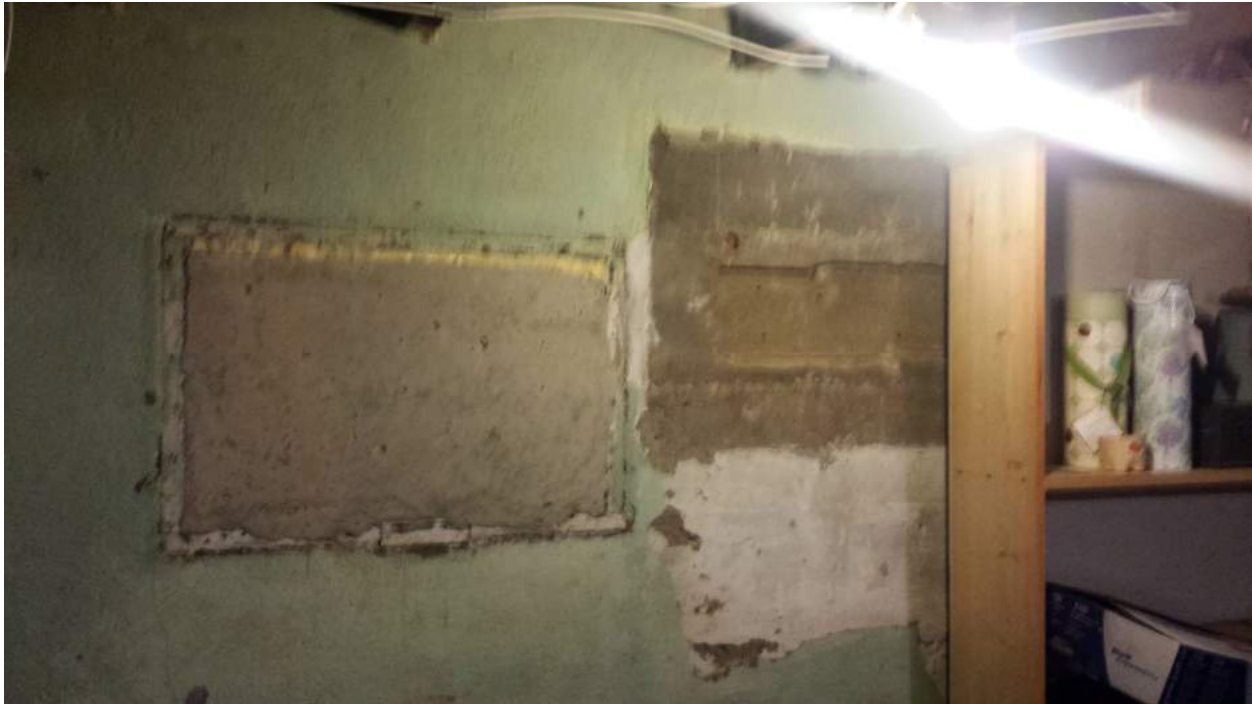
Photograph 7: The basement of 402 Roosevelt Avenue; former window or possibly a former coal chute.
