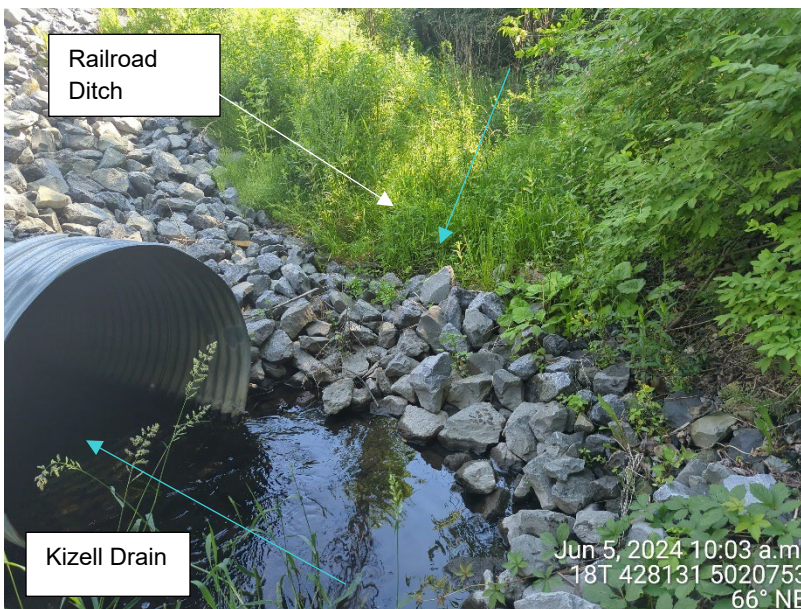
Photo 4: Rip rap at Kizell Drain creating a barrier at the downstream end of the ditch (June 5, 2024)
