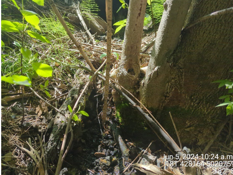
Photo 3: Tree in the channel resulting in steep of 22cm, downstream end of the culvert (June 5, 2024)
