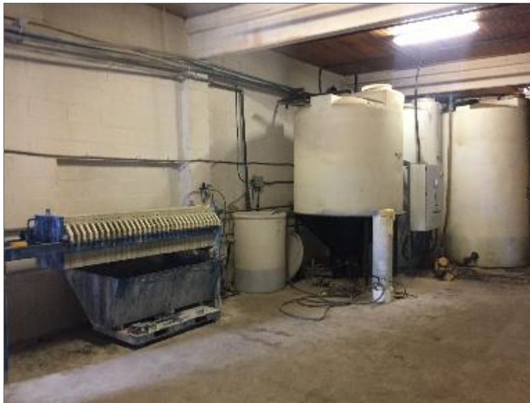
Photo 8 – Three ASTs located within Site Building B that treat the wastewater collected in the trench system/holding tank prior to discharge to the municipal sewer system.
