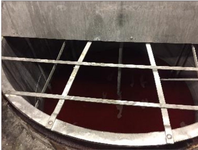
Photo 7 – Holding tank within Site Building B (collection of wastewater from trenches in the manufacturing area).
