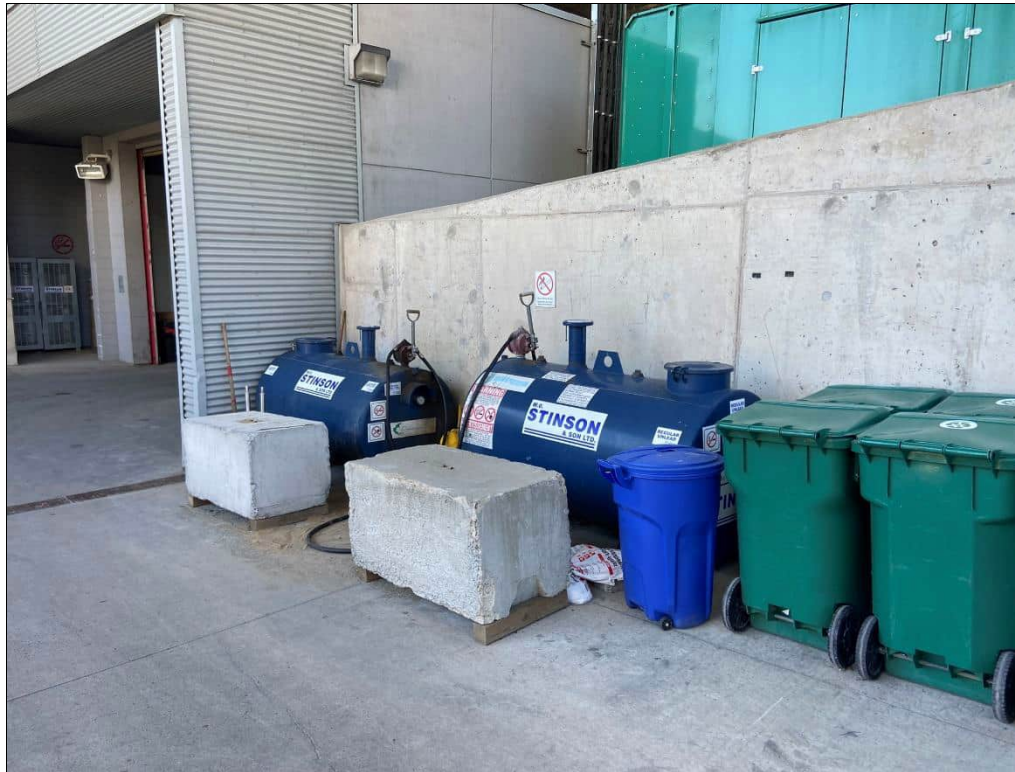
Photo 11: 500 L capacity coloured diesel and gasoline above ground storage tanks located on the ramp outside the loading dock area. Note: fuel spills would flow down the ramp to the grate floor drain. Date: 06/28/24 Direction: Southwest
