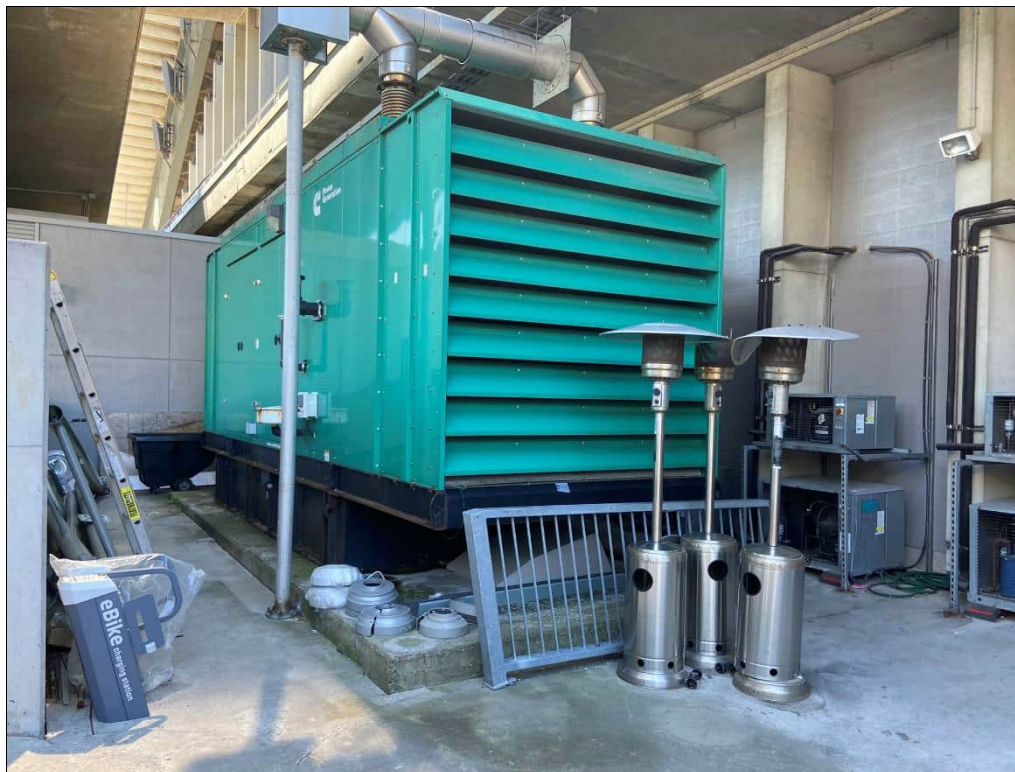
Photo 12: Back-up generator located outside the loading dock area on the east side of TD Place Stadium. Fitted with a 5,791 L capacity diesel storage tank. Date: 06/28/24 Direction: South
