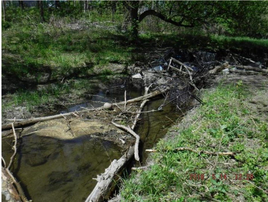
Photo 15: Garbage and debris jam between stations 1 and 2 (May 14, 2018)
