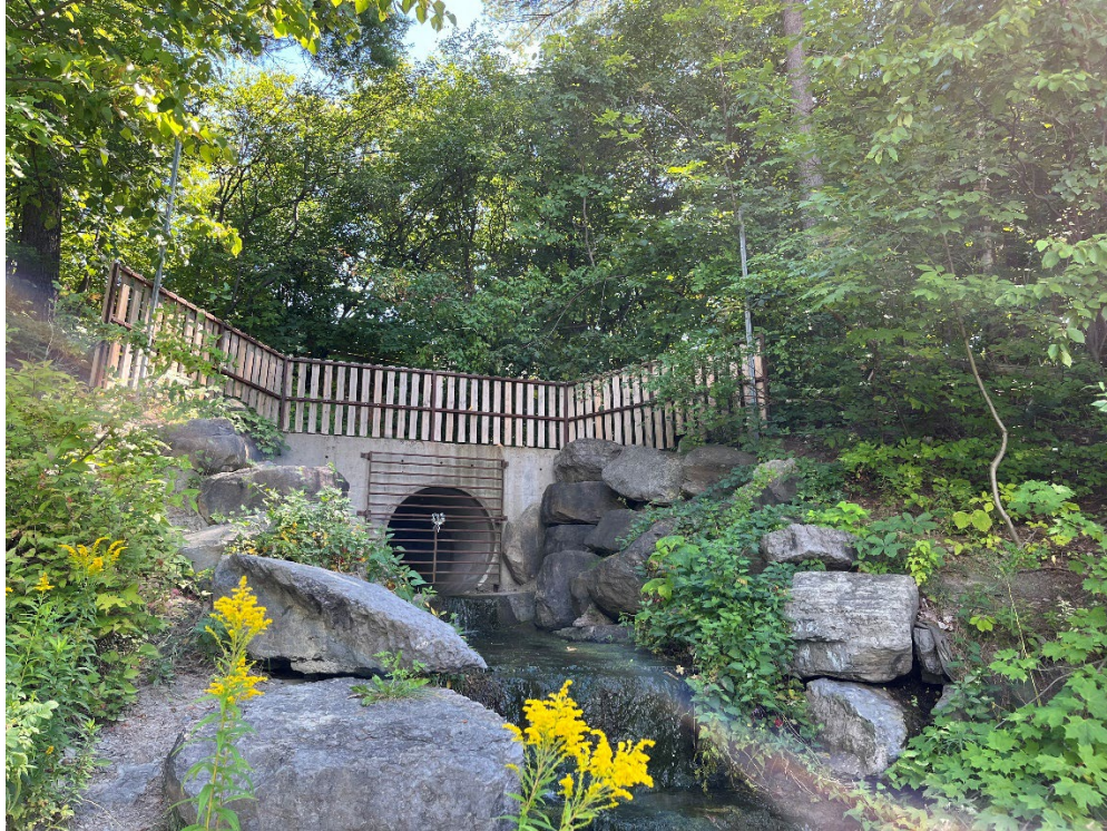
Photo 3. Culvert outlet with discharge onto bedrock at an approximate elevation of 80 m (see Figure 02). Photo taken by BGC 2022-08-15.
