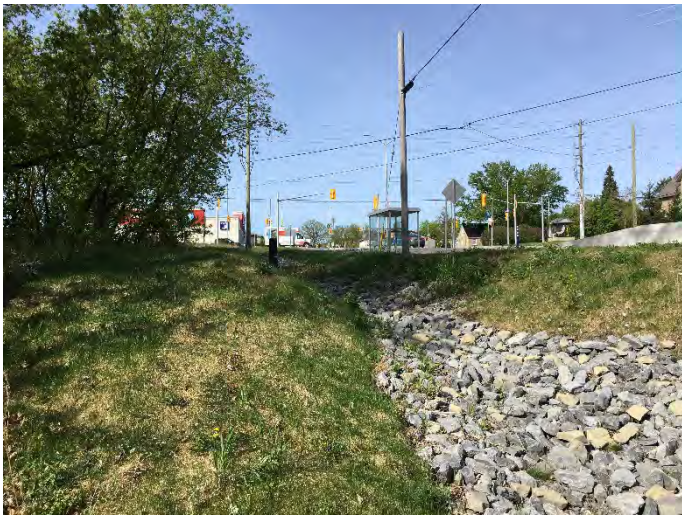
G – Drainage swale with rip rap, northern boundary of site along Klondike Road, looking southwest
