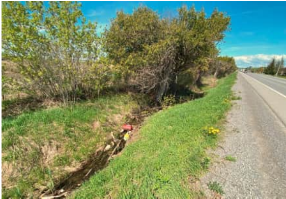
PICTURE 3: Example of Minor Debris Buildup - Facing Northwest
