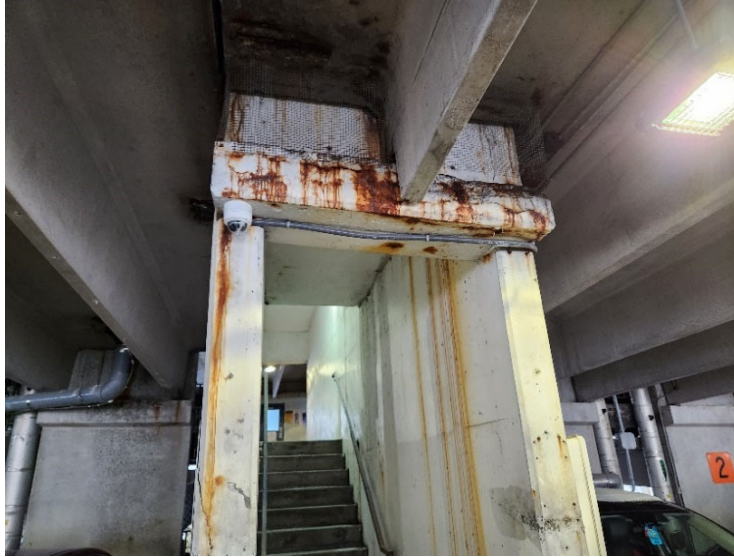
Photo 15 - Rust staining on stairwells
