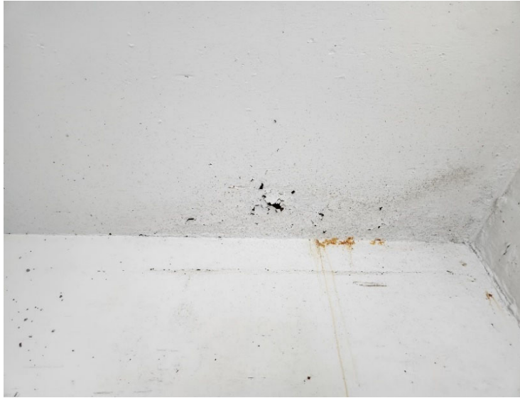
Photo 11 - Peeling paint in stairwell
