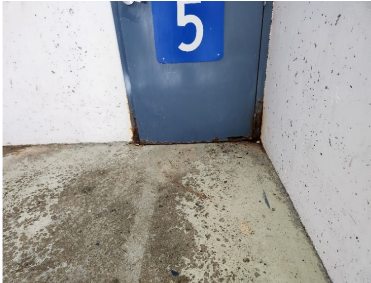
Photo 12 - Rusting/corroding door frame
