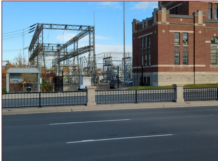
Photograph 7: Power Station at 1275 Carling Avenue.
