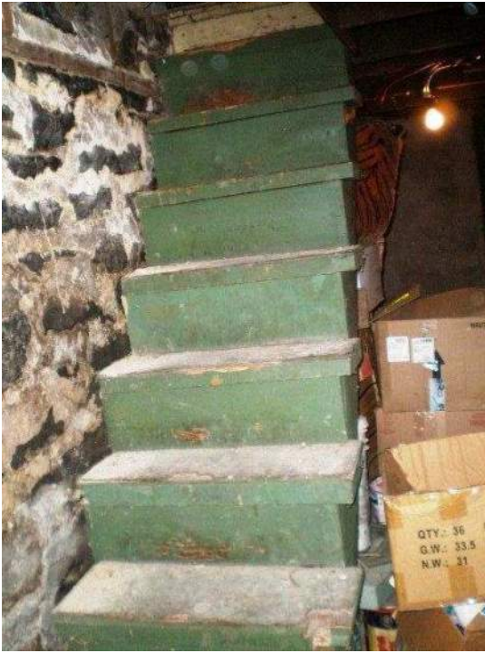
Missing interior handrail
