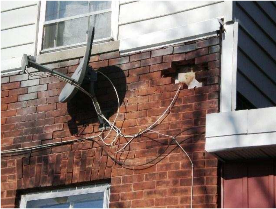
missing bricks on ext. wall
