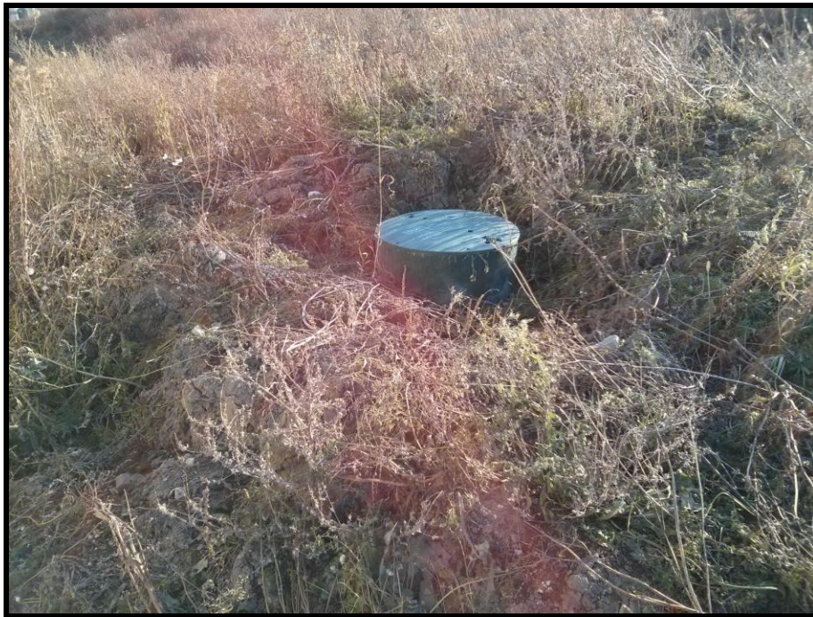
Photograph 4: View of the sewage holding tank on the eastern portion of the property.
