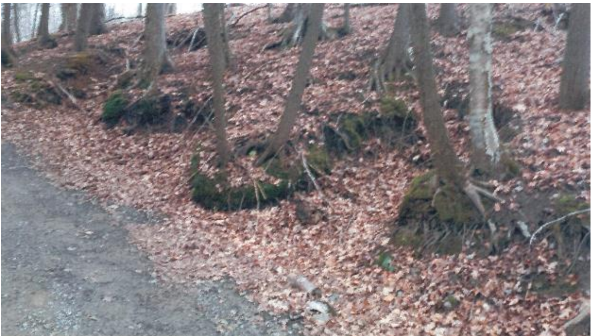
Photo No. 10 – Erosion of cut uphill of pathway. Cut approximately 20 m long x 0.4 m to 1.2 m high.
