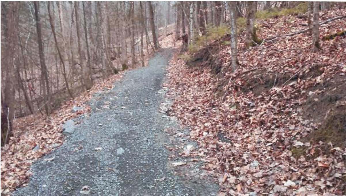
Photo No. 21 – Erosion of cut above pathway. Cut approximately 45 m long x 0.3 m to 0.8 m high.
