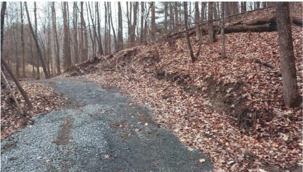
Photo No. 2 – Erosion of cut uphill of pathway. Cut approximately 9 m long x 0.4 m high.
