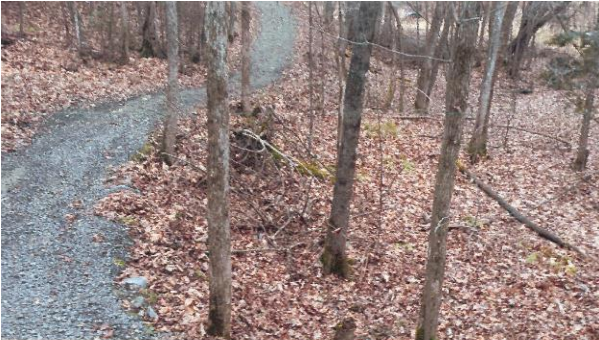
Photo No. 20 – Deep cut downhill of pathway. Cut approximately 12 m long x 0.5 m to 1 m high.
