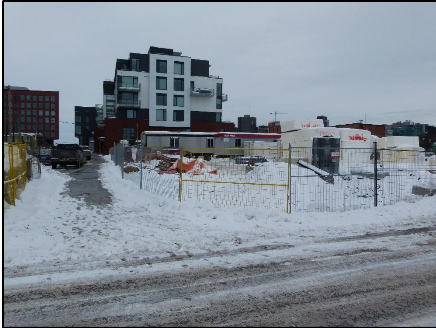
Photograph 3: Looking east at the materials storage and site trailers within the southern part of the Site. The recently constructed building in Block 205a is visible in the background (February 4 th , 2022).
