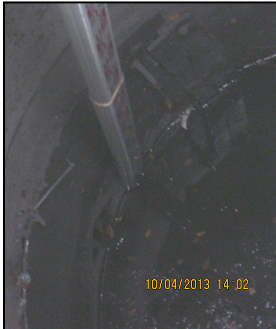
Figure 2a: Gate/Orifice in MH16
