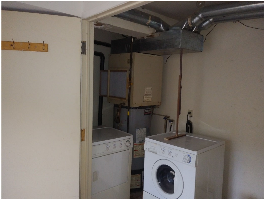
Photograph 8: View of one of the ground floor mechanical rooms in the residential building at the Phase One Property.
