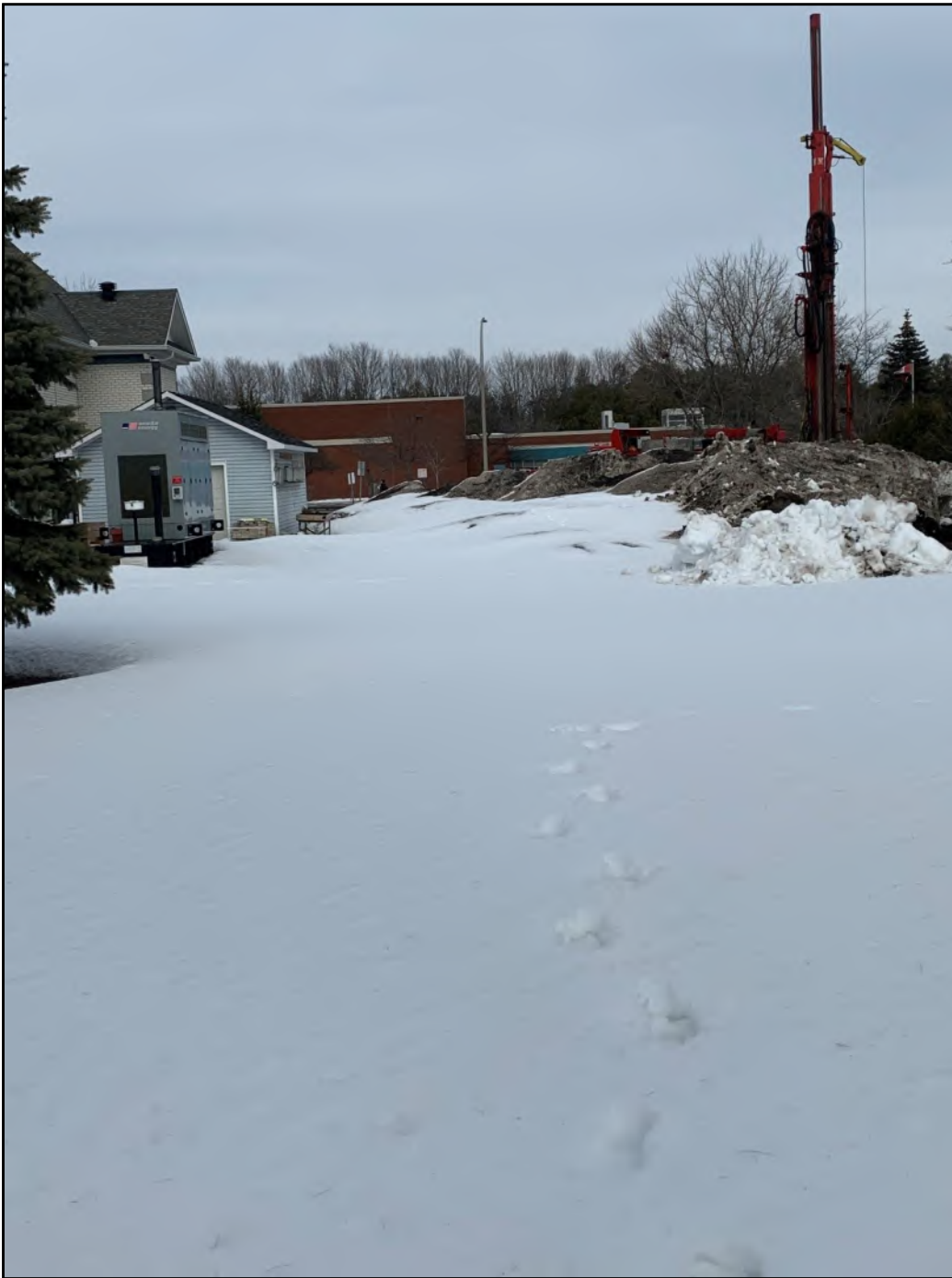
Site Photograph 5: 1364 Stittsville Main Street looking northeast from the back of the Site towards Stittsville Main Street (March 16, 2022).
