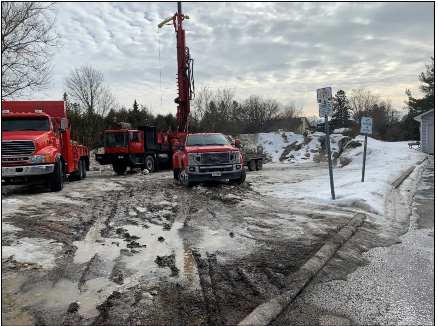
Site Photograph 4: 1364 Stittsville Main Street looking southwest into the Site from Stittsville Main Street. Drilling operations ongoing for the installation of a geothermal well (March 16, 2022).
