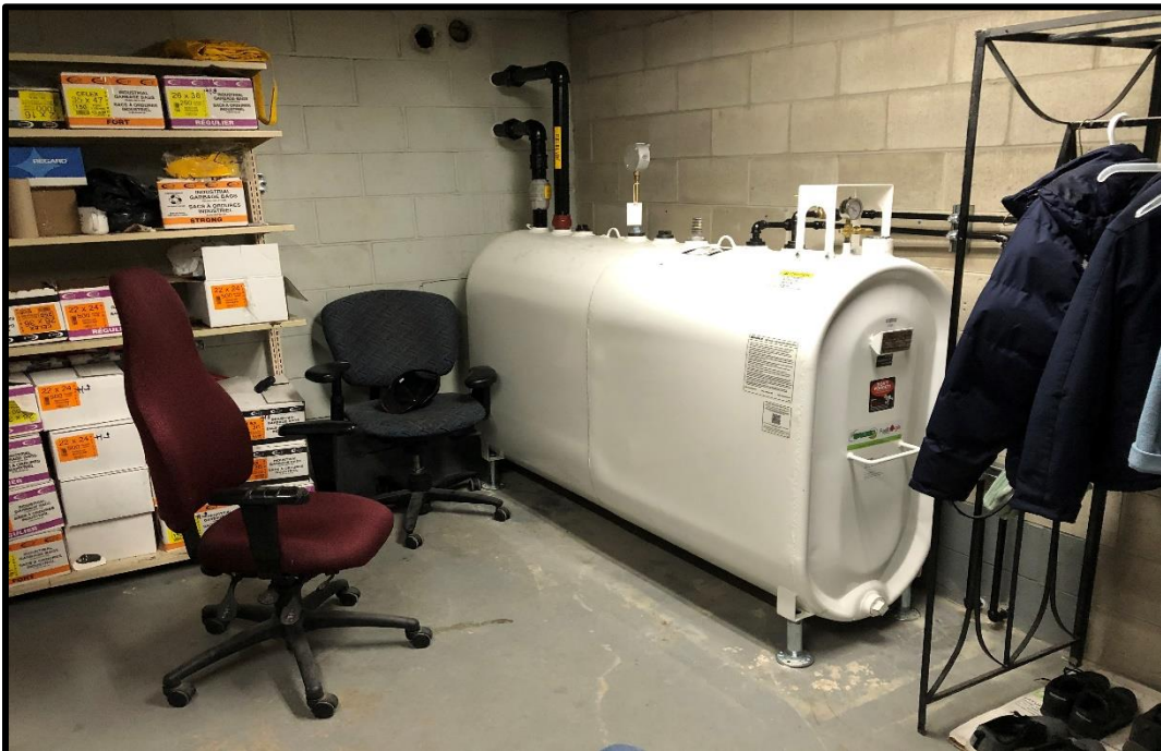
Photograph 4: View of the interior aboveground diesel fuel storage tank, located in the second to lowest basement level of the subject building.
