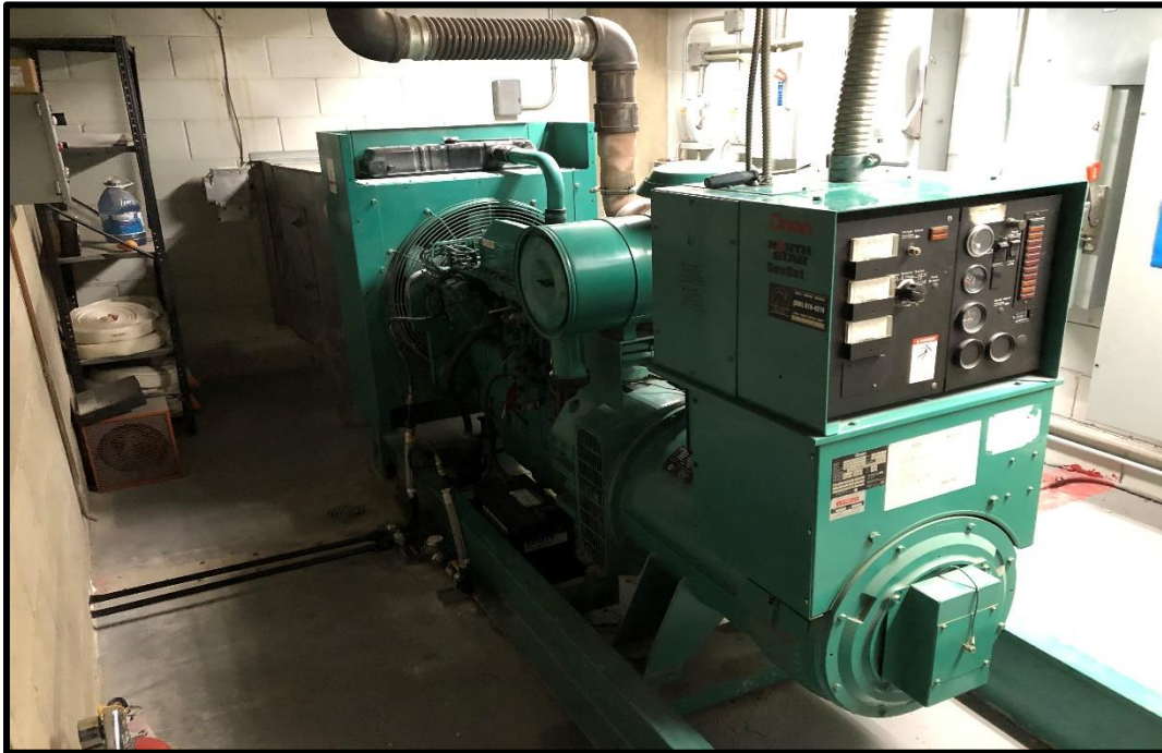
Photograph 5: View of the interior diesel-powered generator, located in the second to lowest basement of the subject building.
