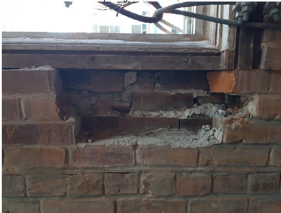
Photograph 12: View of the middle wythe condition. Mortar in poor condition and some cracked bricks. Opening on north wall, second floor (below window to extract middle wythe).
