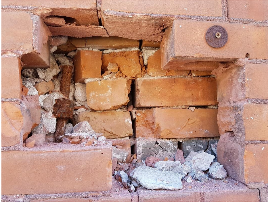
Photograph 13: View of the middle wythe condition. Mortar deteriorated, crack and crushed bricks. Opening on the exterior, ground floor of the north elevation.
