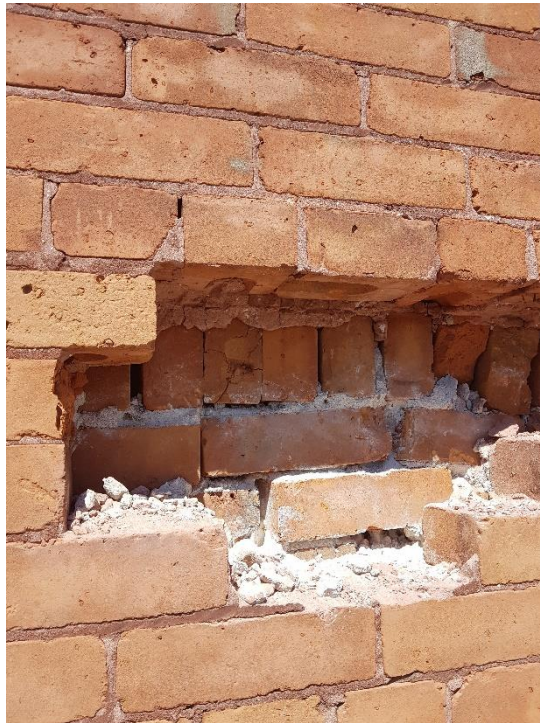
Photograph 11: View of the middle wythe condition. Mortar in poor condition and some cracked bricks. Opening on south wall, third floor.
