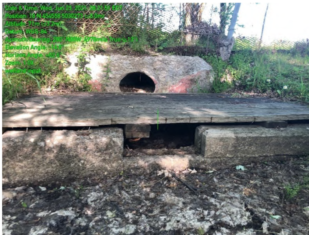
Figure 8 Photo showing the remnants of a dike in the northwestern portion of the wetland on Site (taken June 23, 2021)
