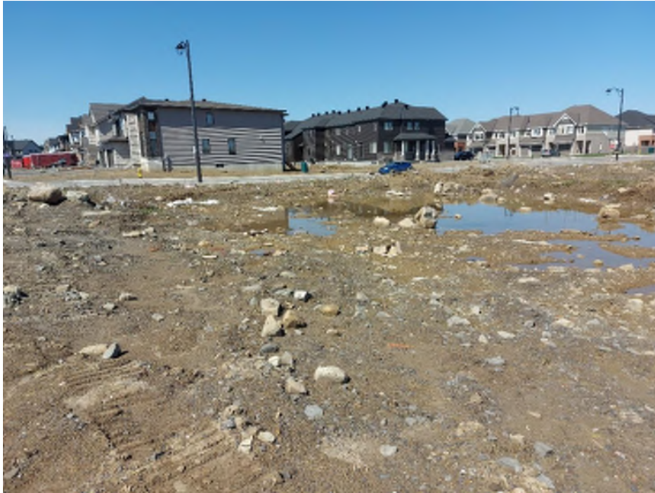
Photograph 1: Onsite cobbles and boulders
