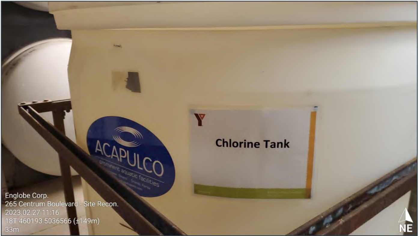
Site Photograph 7: Overview of the plastic chlorine tank (empty) in the pool valve room (basement).
