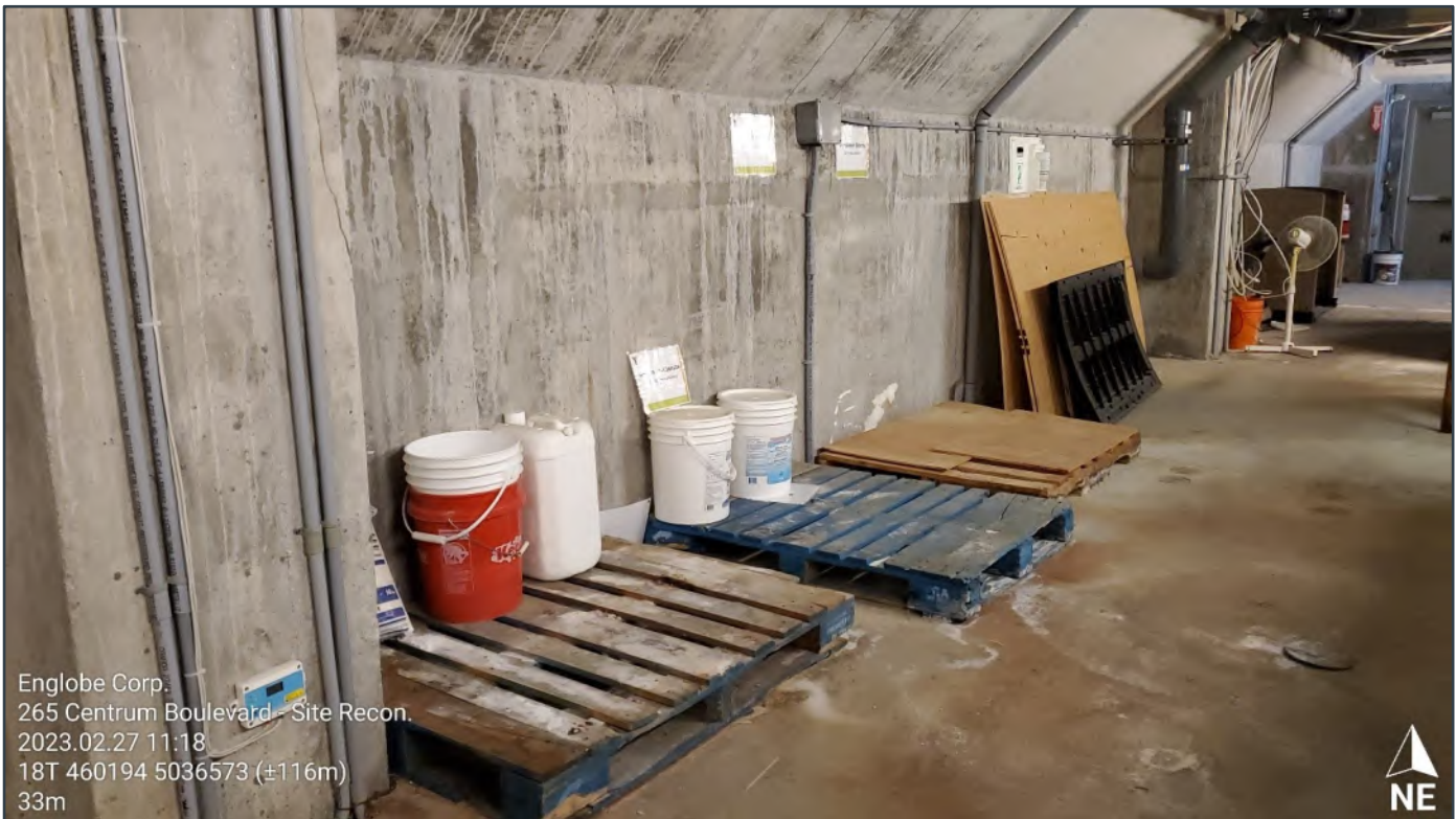
Site Photograph 6: Overview of the pool chemical storage area in the pool valve room (basement).
