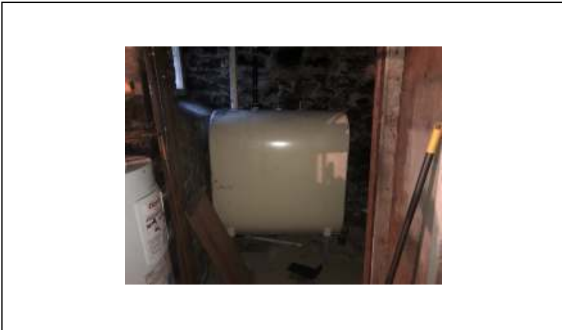
Photograph 13: 680 liter fuel oil above ground storage tank in basement of 12 Hawthorne.
