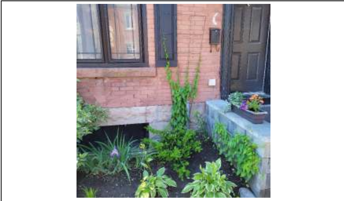
Photograph 5: Looking south at north front wall of 18 Hawthorne, note fill and vent pipes for AST in basement of unit.
