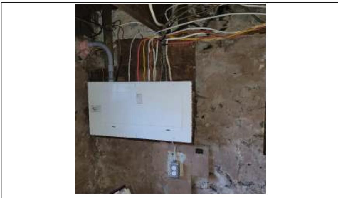
Photograph 24: Main electrical panel in north-east corner of basement of 18 Hawthorne.
