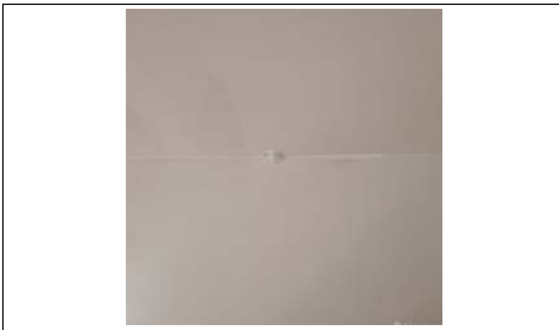
Photograph 9: West wall and ceiling of kitchen in 14 Hawthorne, note main sewer drain in corner of wall/ceiling.
