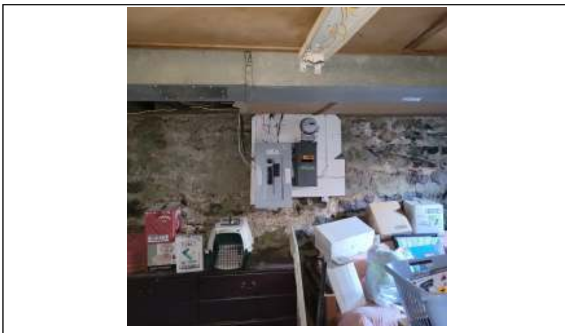
Photograph 10: Main electrical panel in basement of 12 Hawthorne.
