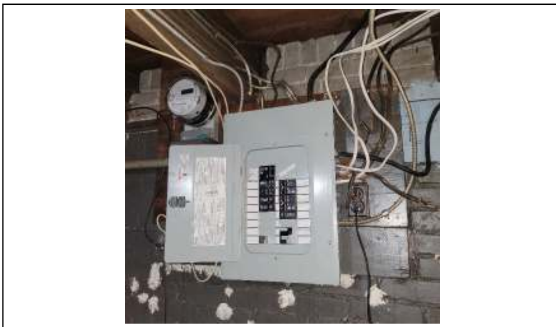
Photograph 7: Main electrical panel in basement of 14 Hawthorne.
