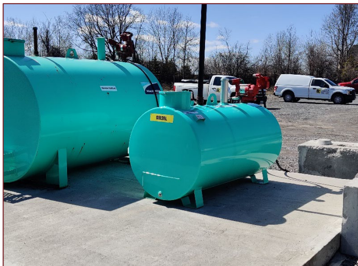
Photograph 5 – Two aboveground storage tanks along the southeast property boundary of Site.
