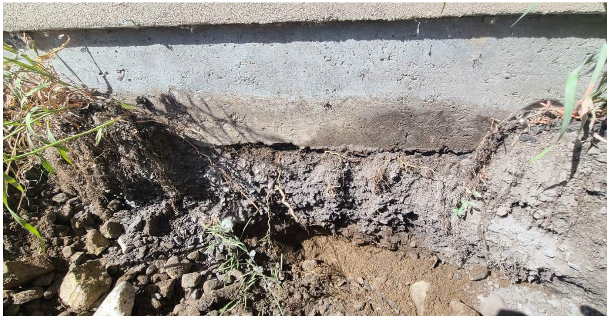
Photograph No. 2: Detailed view of thickened structural slab and subbase materials in Test Pit No. 1
