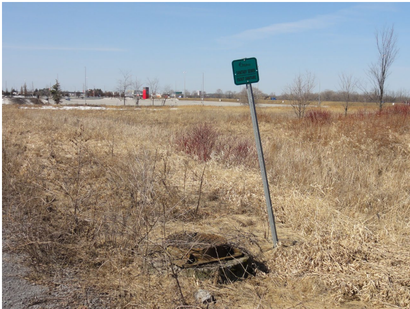
Photo 6 – View of sanitary and storm connections, along the walkway on the central portion, servicing the Site.
