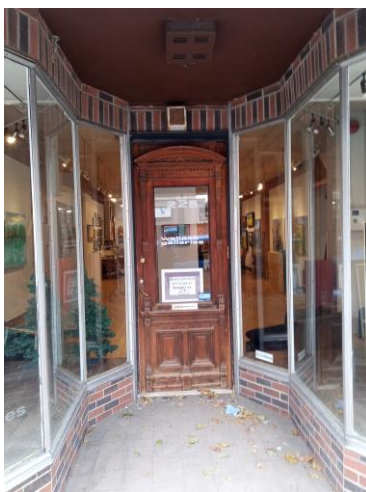
Figure 18: Although the shopfronts have been dramatically altered elements such as the recessed shopfront at 227 Bank Street are still evident. The leaded transom and vaulted arch have been covered over. Based on the 1950 photo it would appear that the three shopfronts at 215, 217 and 219 were similar with recessed entrances and decorative transoms.
