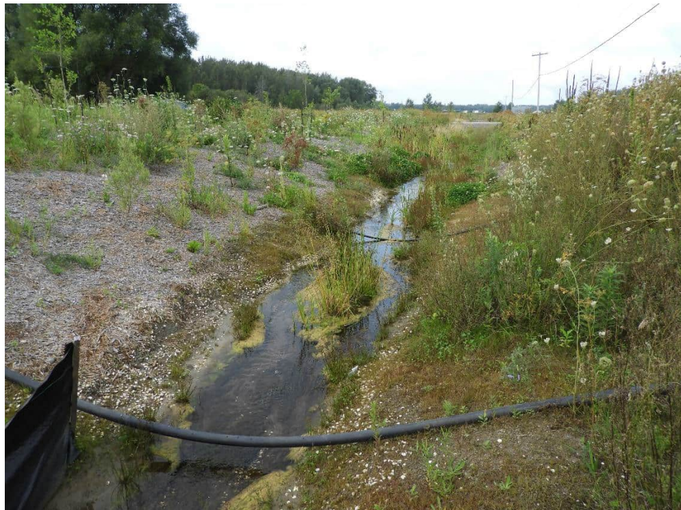
Photo 4: Upstream view of the tributary of Carp River (looking southwest) which was realigned parallel to the south side of Russ Bradley Road (to the right of the photo). 11 August 2021.
