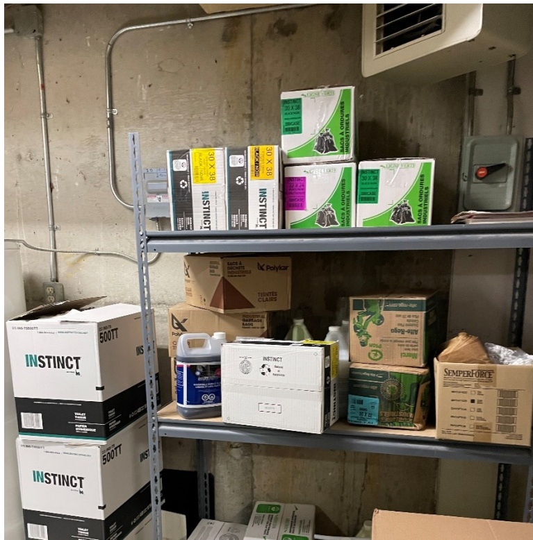
Photo 115: Cleaning supplies in air handler room
