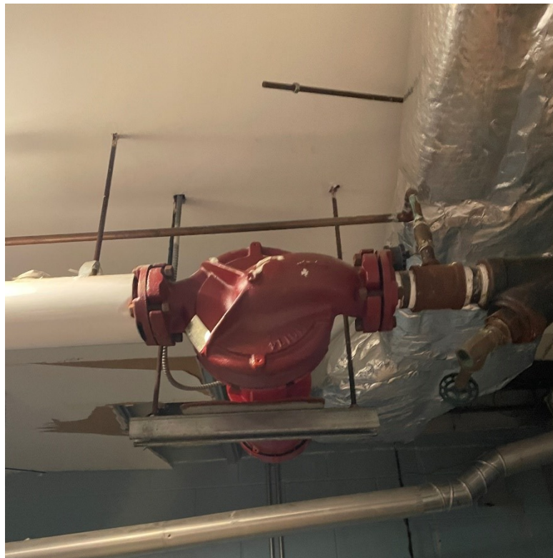
Photo 20: Cause of historic leak in boiler room - has been rectified and no more leaks have been detected
