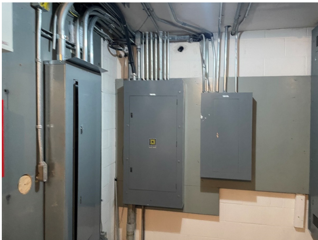
Photo 112: Electrical panels in air handler room
