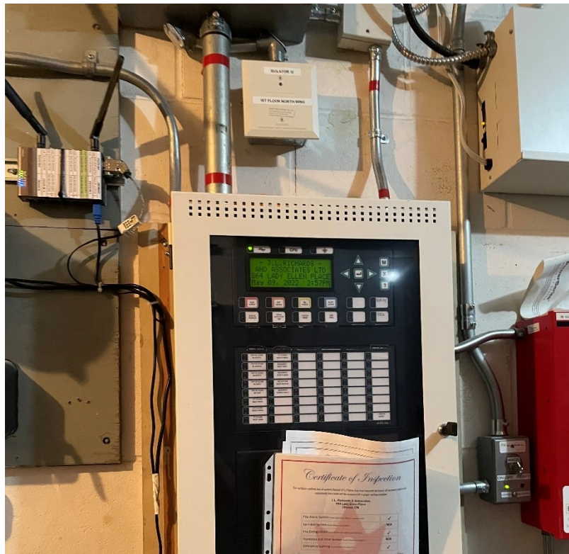
Photo 111: Electrical panels in mechanical room
