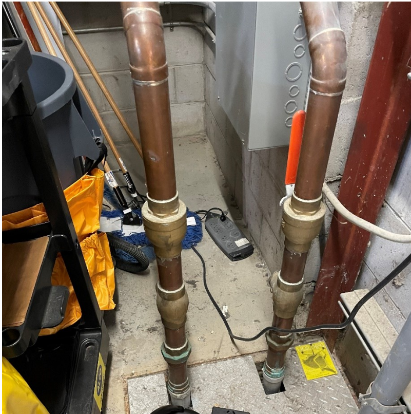
Photo 113: Sump pit with two pumps in air handler room
