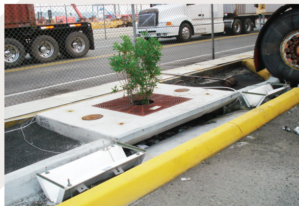
Filterra™ monitoring unit at a port.
