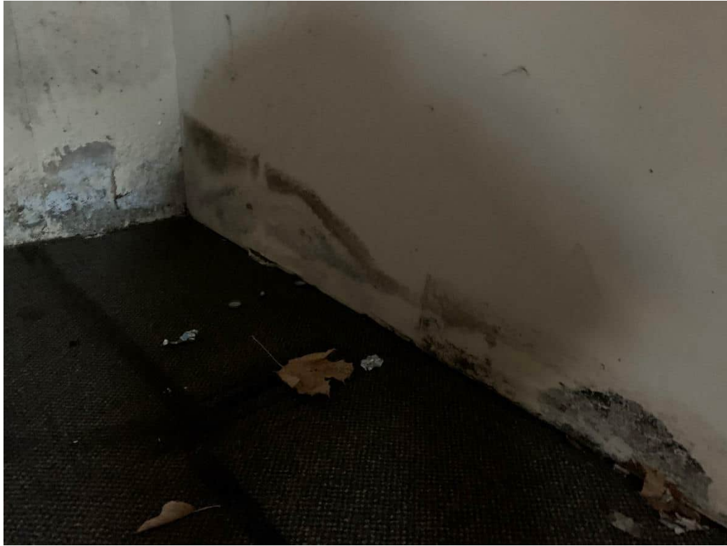
Photo 7: Suspect mould located on the dry wall within the basement level of the Site Building.
