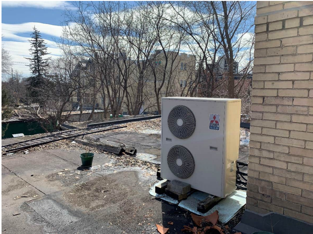
Photo 8: Roof-top split-level air-conditioning unit for the Site Building.
