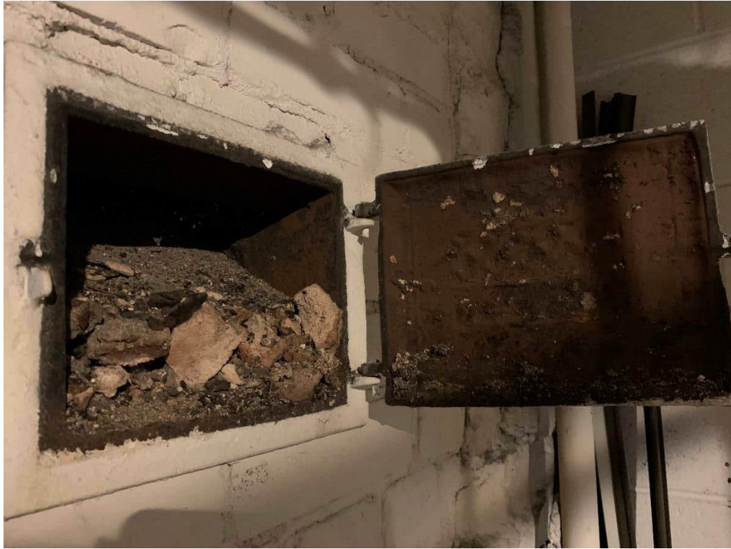
Photo 5: Garbage incinerator located within the boiler room of the basement level within the Site Building.
