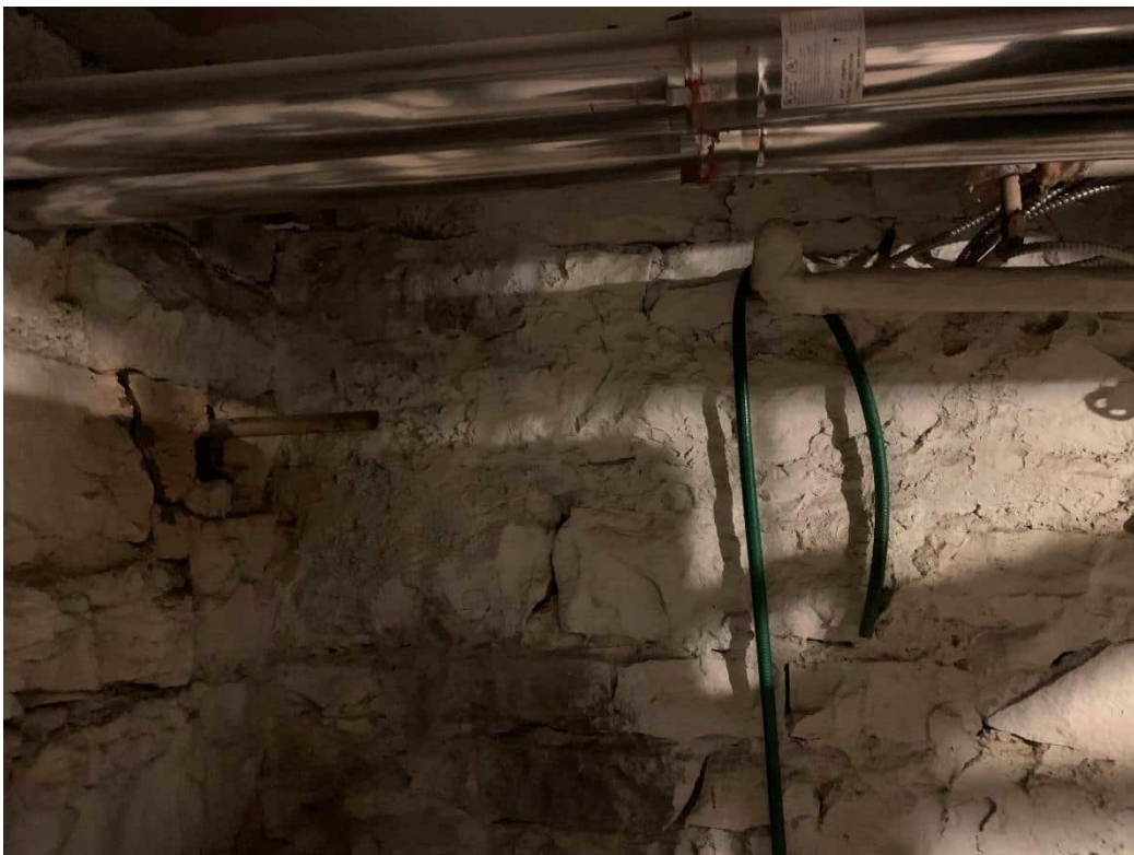
Photo 4: Piping from suspected aboveground storage tank within the basement level boiler room of the Site Building.
