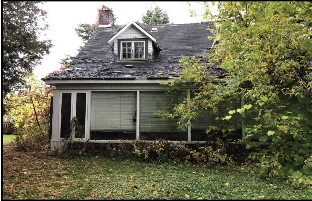
Photograph 3: View of the abandoned residential dwelling situated at 741 Blair Road, facing west.
