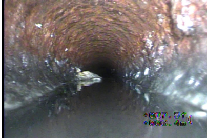
Figure#9: A view to the diameter change to 150mm and 12 o'clock connection at 9.8 meters from the top of floor CO.
