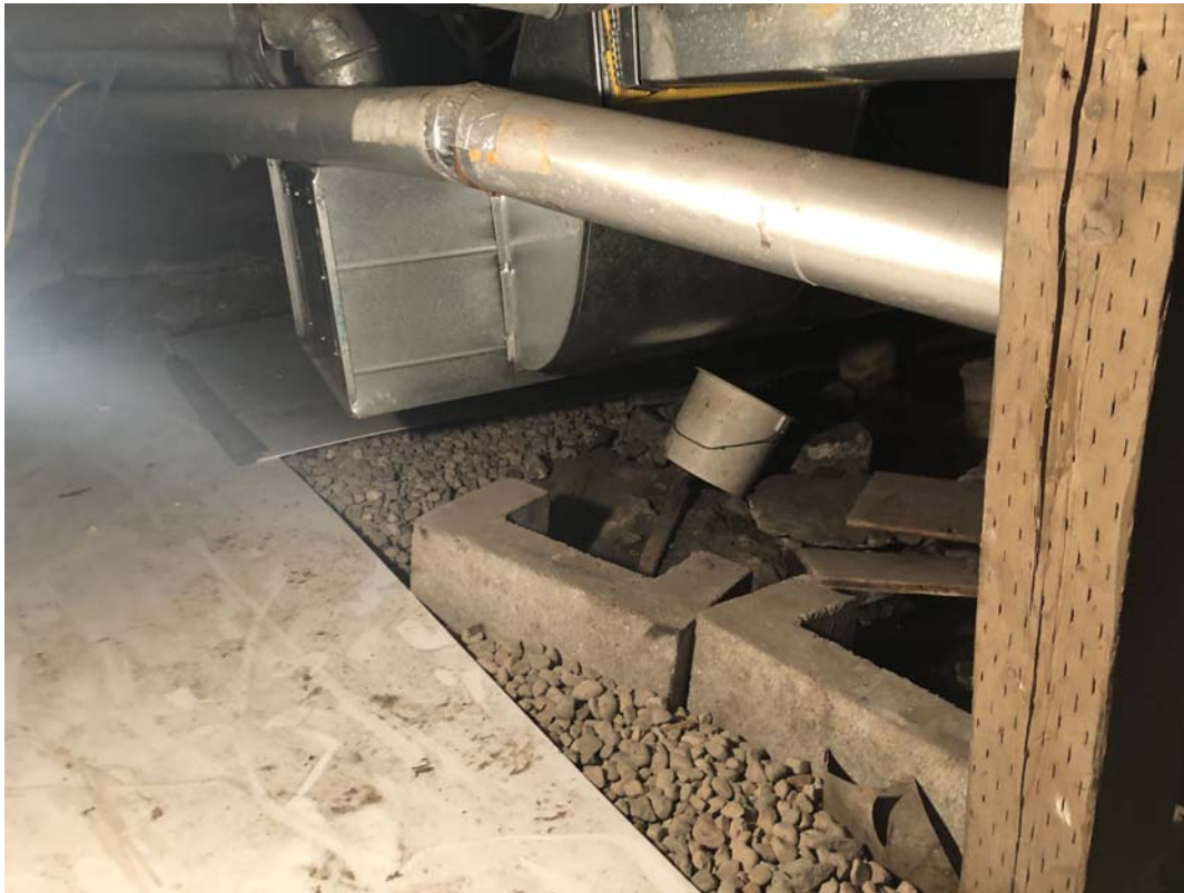
View of furnace with basement crawl space.
