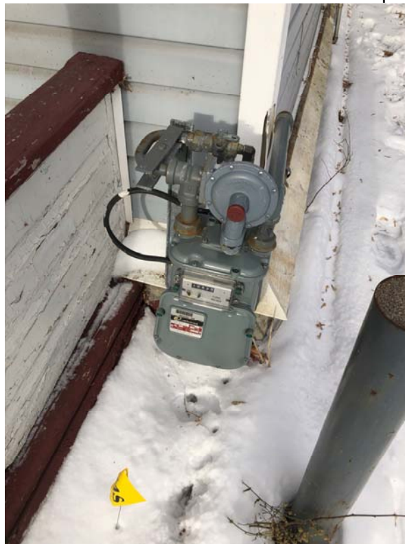
View of natural gas meter servicing site.
