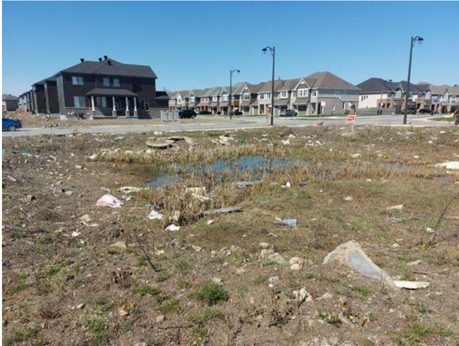
Photograph 5: Low lying area of poor drainage
