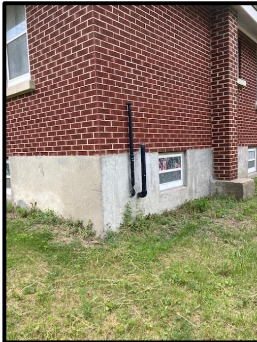
Photograph 2: View of vent and fill pipes at the back of 98 Bearbrook Road, facing southeast.
