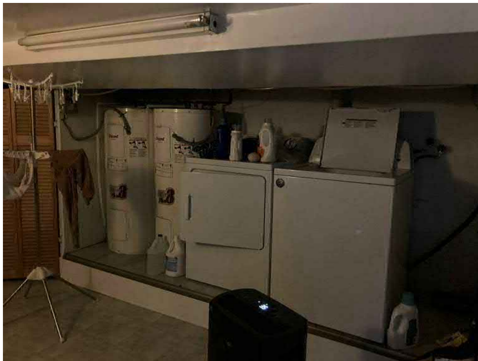
Photo 4: View of the laundry room in the basement of the building.
