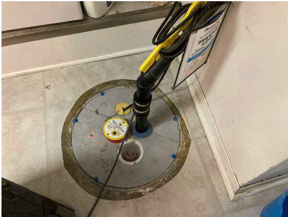
Photo 5: View of the sump pump located in the laundry room of the basement.
