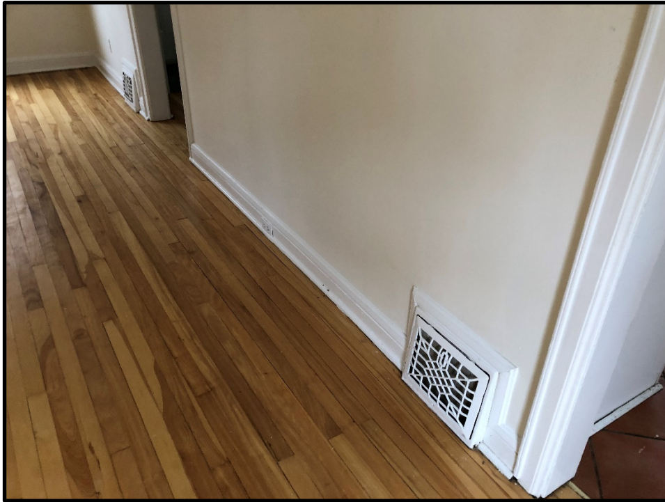
Photograph 1: Floor and walls of the first-floor living room.
