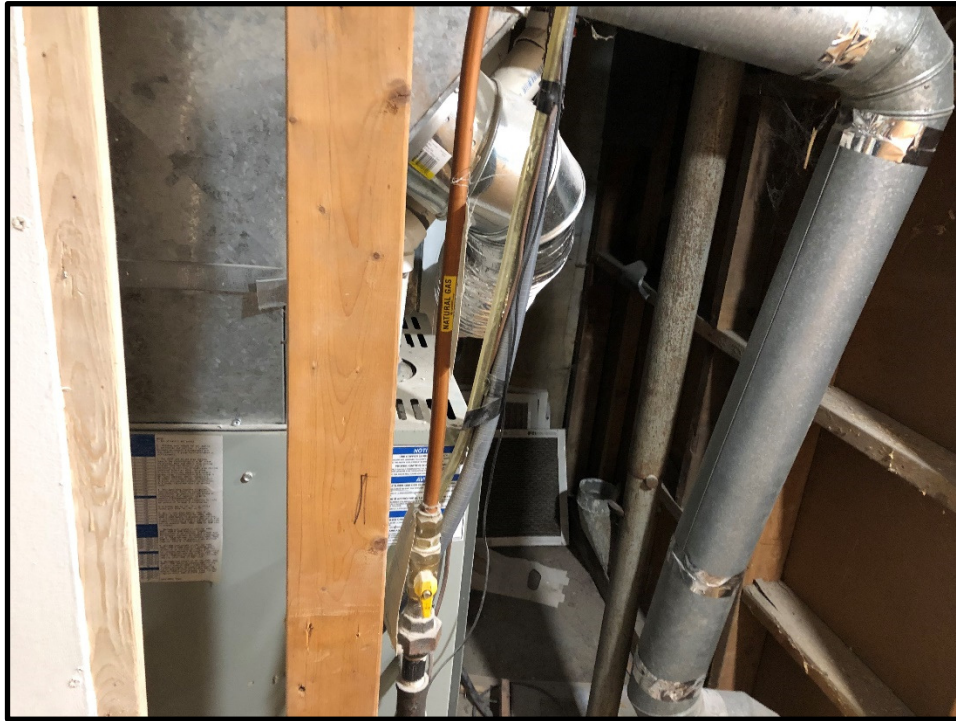
Photograph 3: Natural Gas furnace located in the basement of the property.
