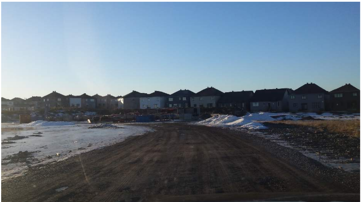
Photograph 4: Construction site office and storage area south of Russet Terrace, looking north.
