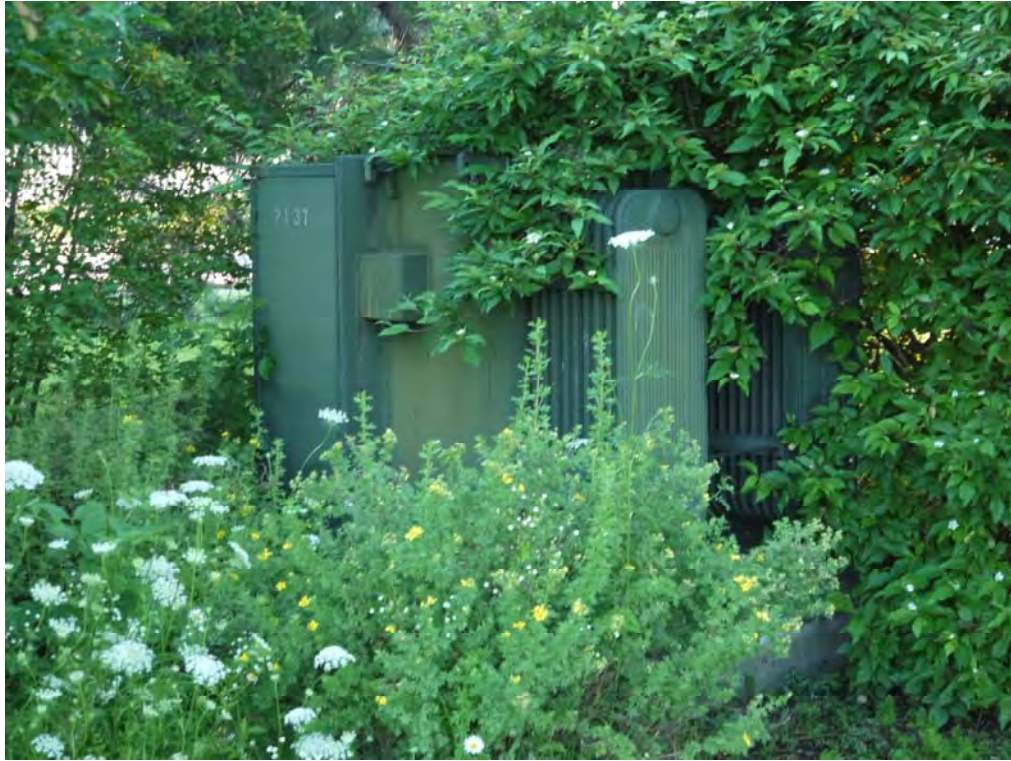
Transformer adjacent to northeast corner of site (located at 2355 St Laurent Boulevard) with possible PCB containing equipment.
